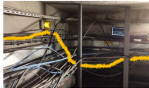
(a) Location of the measure and position of the deployed fiber cable in tunnel (highlighted cable)
